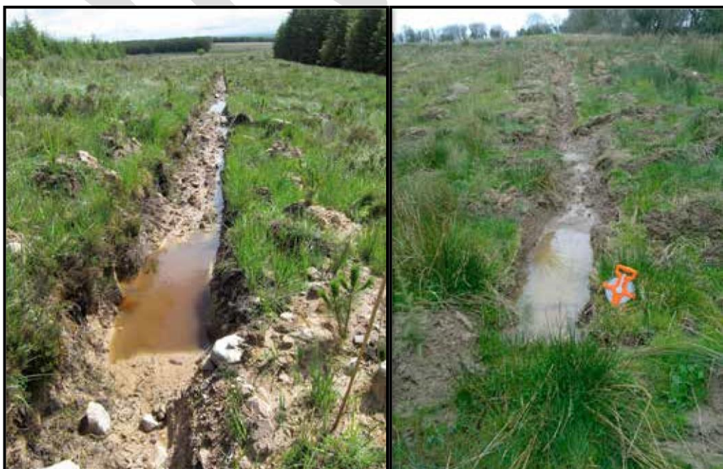
Figure 9.2 In-drain sediment trap (left) and a sediment trap adjoining a water setback (foreground) (right).
